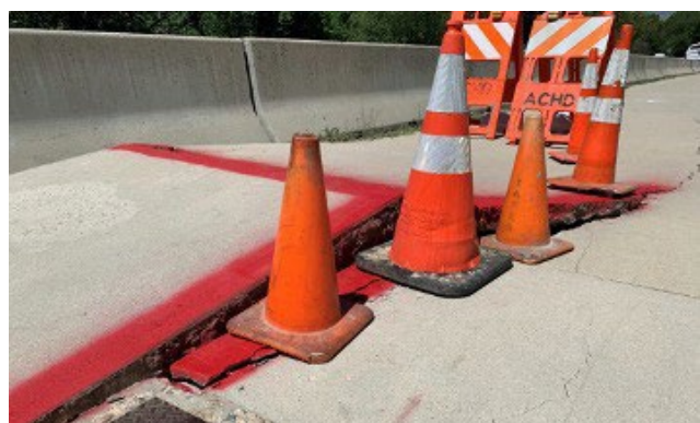
Figure 1. Heat-related pavement buckle on Veterans Memorial Parkway in Boise. Photo: Ada County Highway District.
